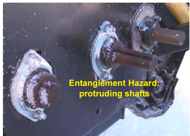
Figure 7. Protruding shafts with keyways are potential entanglement hazards.
