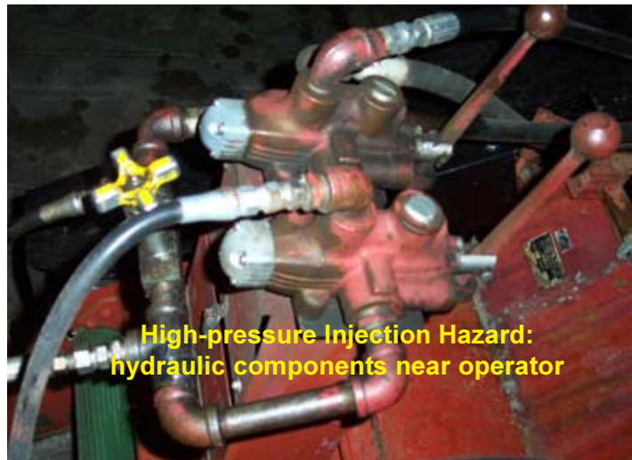
Figure 17. Pin hole hydraulic leaks are a hazard to the skin and eyes.
