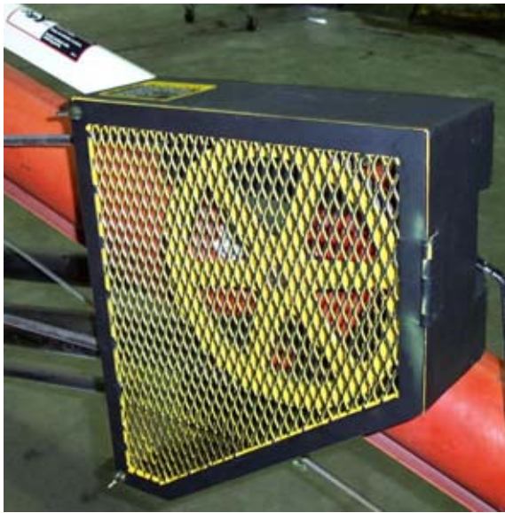
Figure 50. The driven pulley guard.
