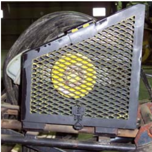
Figure 45. Driven pulley completely guarded.
