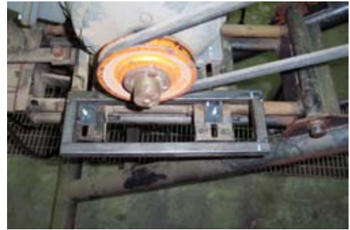
Figure 48. The guard frame bolted to the motor mount frame.
